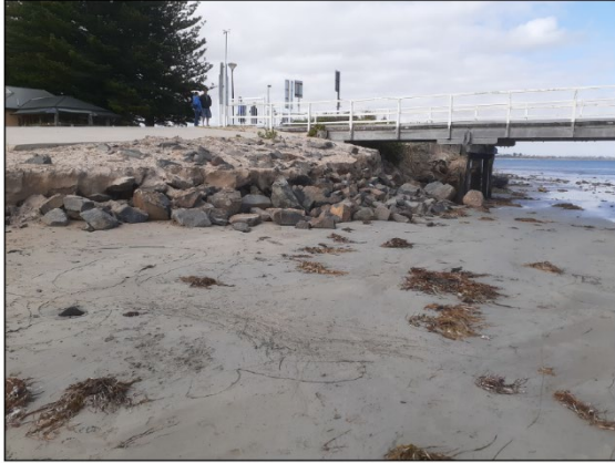
November 2019 Storm damage next to the causeway
