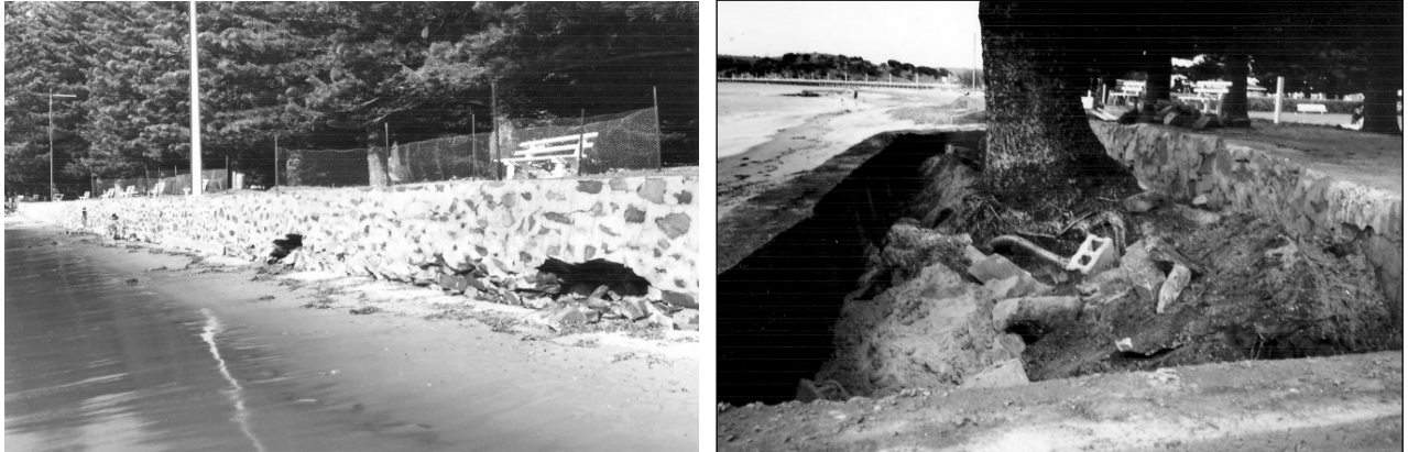
Figure 18. The seawall was undermined and repaired in 1975. The Norfolk Pine was retained by 'boxing out' the wall.
