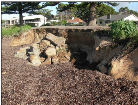
June 2014 Opposite house numbers 74/75. Erosion very close to the footpath
