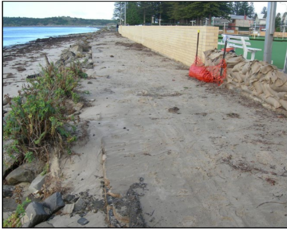
June 2014 The Bowling Club wall was damaged and had to be rebuilt after a storm
