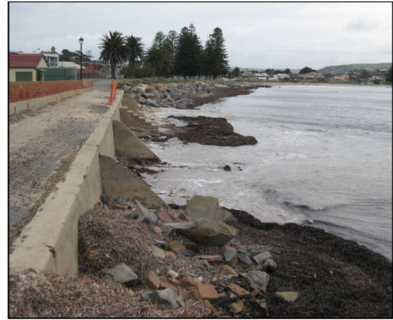
October 2009 Bowling Club showing severe erosion back to foot path wall and showing old red brick wall prior to the construction of the yellow wall.
