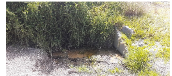
Figure d. Fell Street outlet. Same location as Figure (a). The headwall tends to prevent undermining from actions of the sea.
