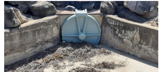
Figure a. Headwall tends to prevent undermining from actions of the sea.
