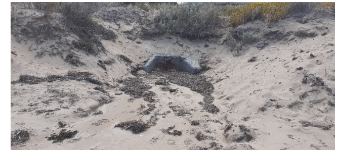
Figure b. Some outlets require maintenance (not the focus of this assessment)
