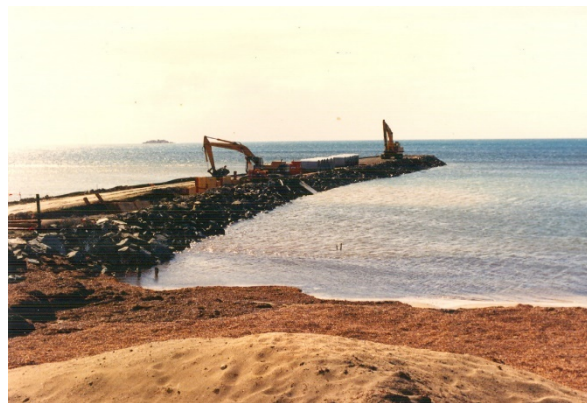
Figure a. Installation of pipe to ocean floor by way of temporary rock and earthen structure, pipe installed in the middle (Photograph - Coast Protection Board, 19860319).
