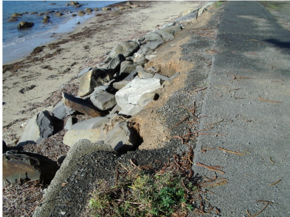
Figure a. Erosion damage near Nevin Ave, 3 August 2004, 1.925CD (Photograph - Coast Protection Board, 20040810).
