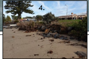
4. Rock revetment (buried in embankment) – poor condition.
