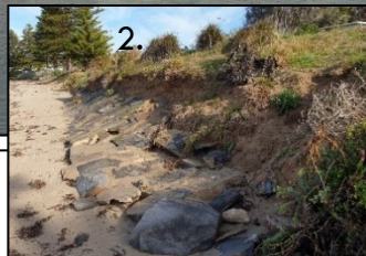
2. Rock and concrete seawall – installed in 1950s (condition poor)
