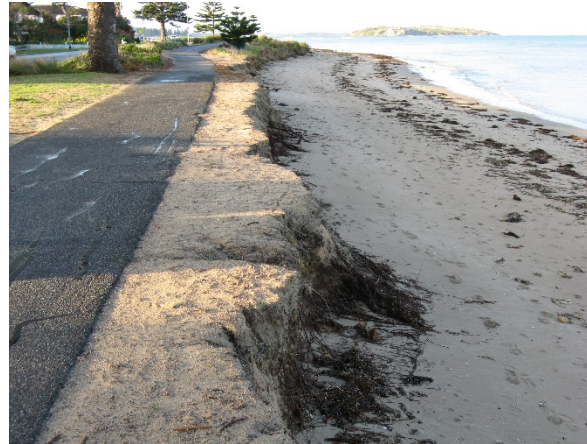
Figure c. Erosion damage between Fell Street and Fountain Ave, June 2011 (Photograph - Coast Protection Board, 20110616).
