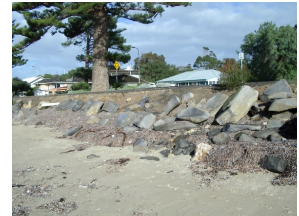
Figure c. Erosion damage near Nevin Ave, 3 August 2004, 1.925 CD (Photograph - Coast Protection Board, 20040810).
