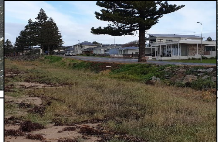
3. A gap in the protection works – but not under immediate threat.
