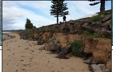
4. Rock revetment – recently eroded so that rocks are sliding on to the beach.
