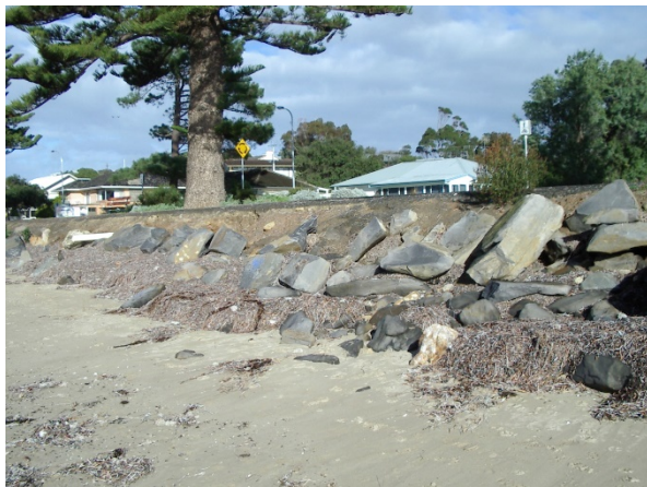
Figure b. Erosion damage near Nevin Ave, 3 August 2004, 1.925 CD (Photograph - Coast Protection Board, 20040810).
