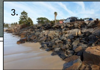
3. Rock revetment – in poor condition. Install date unknown.
