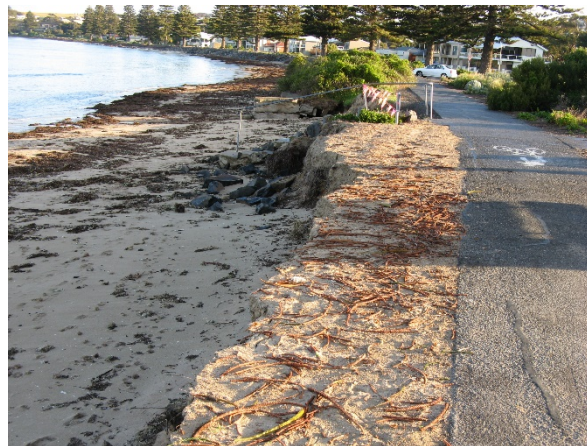
Figure d. Erosion damage between Fell Street and Fountain Ave, June 2011 (Photograph - Coast Protection Board, 20110616).
