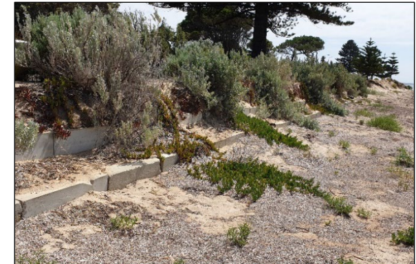
Figure c: Concrete block seawall installed as a trial 5 tiers high, covered with sand and vegetated in the region of Fell Street.
