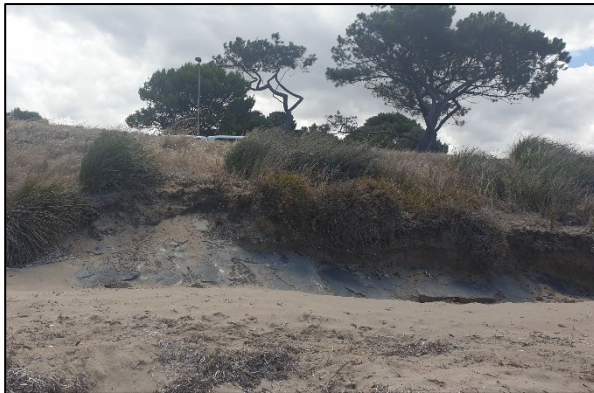
Figure a. Franklin Parade (Yilki). A sloping stone wall was installed in this region in 1949-1951. (M. Western, 2021)
