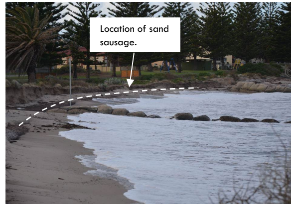
Figure a: Sand sausage installed along the beach near King Street; sandbag groynes installed perpendicular to the beach (CPB, 20120604).
