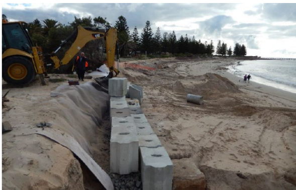
Figure a: Concrete block seawall installed within the dune and covered over with sand (Coast and Marine Branch, email, 2021).
