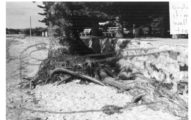
Figures a-b: Damage to seawall – note the intention to retain the tree and to provide a 'planter box' edge (19750101, CPB).
