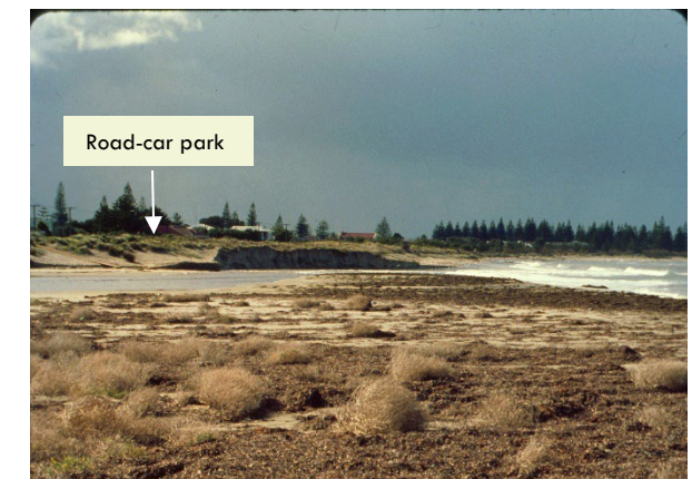
Figure e: Severe erosion of embankment which left unchecked may have threatened road infrastructure on corner of Inman Road and the Esplanade (Photograph: Coast Protection Board, 1 Sept 1979).
