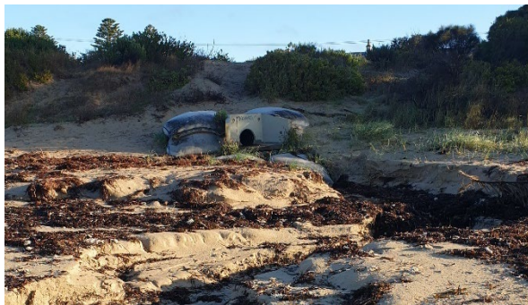
Figure a: Flows from storm water outlets placed at the back of the beach prevent a consolidated and well vegetated dune from being built which could act as a natural defence in the context of rising sea levels.
