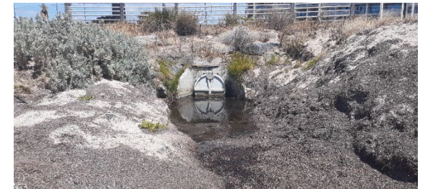
Figure b. Outlets along Flinders Parade are set at very low elevations. Increasing sea levels will increase the times at which these tidal flaps are closed and increase the risk that flooding will be exacerbated within the township.
