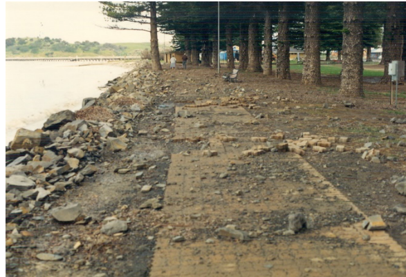
Figure b: Wave over-topping at Soldiers Memorial Gardens (Photograph: Coast Protection Board, 12 September 1989).
