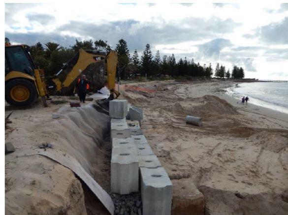
Figure b: Concrete blocks installed in backshore near King Street, covered with sand and vegetated (Email_CMB_20210217).
