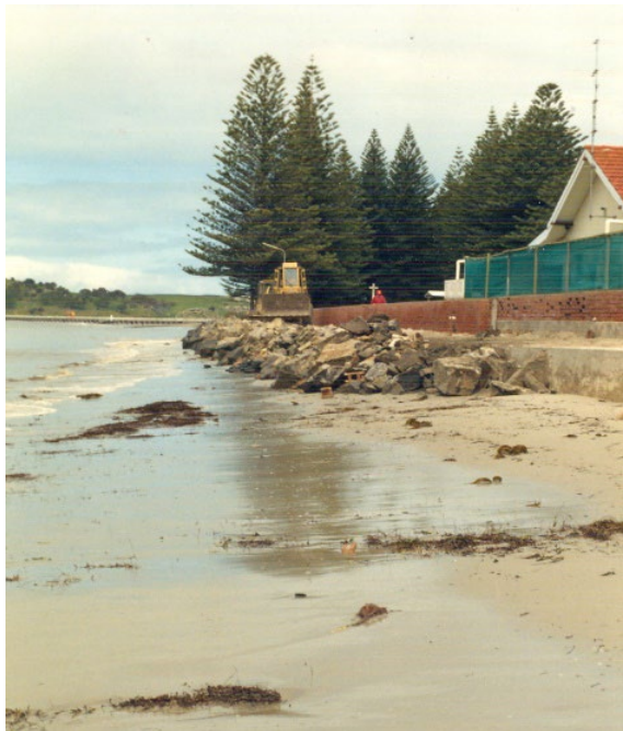
Figure a: Rock protection installed as emergency works after storms of 10-11 September 1989 (19890912, CPB).
