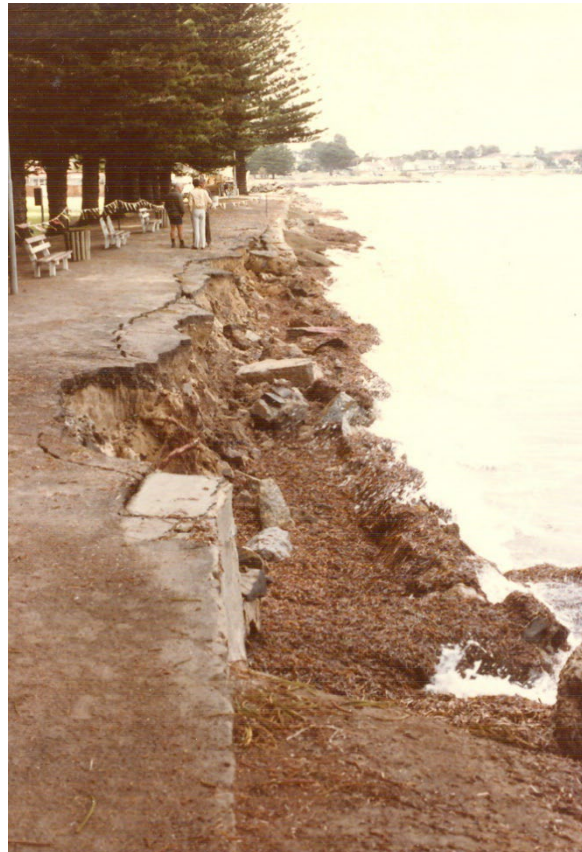
Figure b: Storm event of 17 April 1986 caused collapse or serious undermining of 240m of the seawall (Photograph: Coast Protection Board, 1 May 1986).
