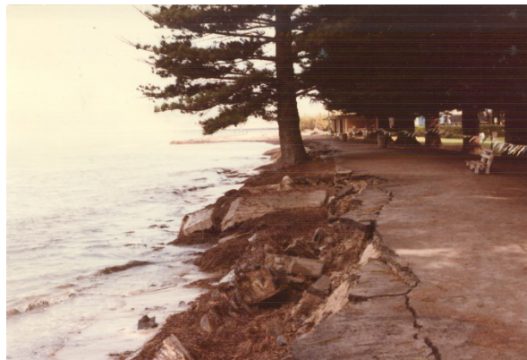
Figure a: Storm event of 17 April 1986 caused collapse or serious undermining of 240m of the seawall (Photograph: Coast Protection Board, 1 May 1986).
