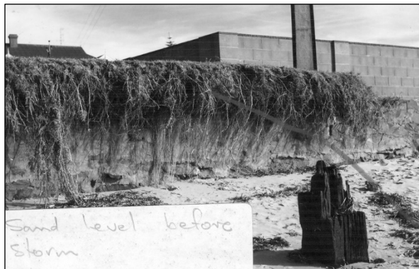
Figures a-b: Damage to seawall – note the drawing on the photograph to indicate the profile of the embankment prior to the storm (19750521, CPB).
