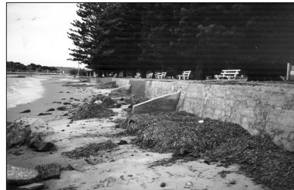
Figures c-d: The seawall was repaired or rebuilt with a section boxed out to maintain the Norfolk pine (19750901, CPB).
