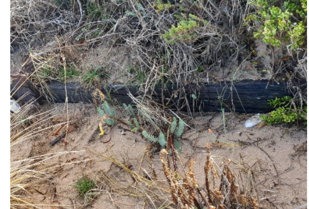
Figure b: Since 1949 the dunes have accreted and most of the retaining wall is buried.
